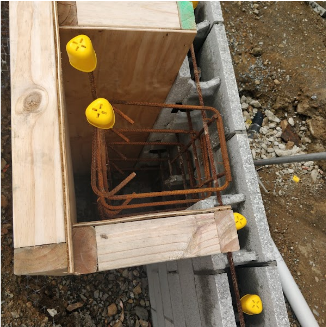
29/11/2021 10:00:00 AM Masonry block column - 4/HD16 with R10-200 ties. Location as per plan
