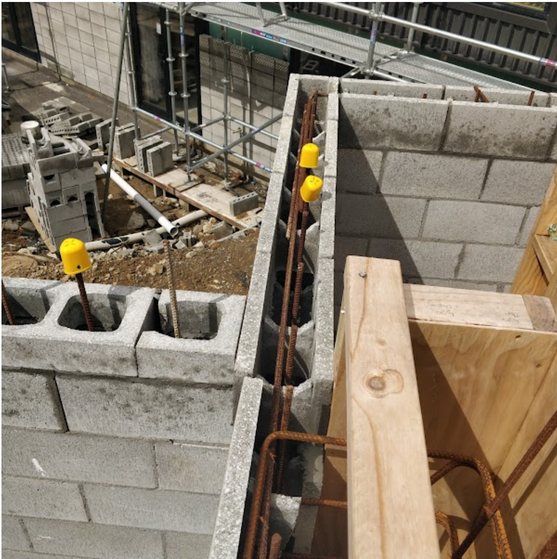
29/11/2021 10:00:00 AM Corner junction to be amended. Details to follow Typical T-Junction as per approved consented plans (refer to General Notes). Photos to be supplied by the builder.
